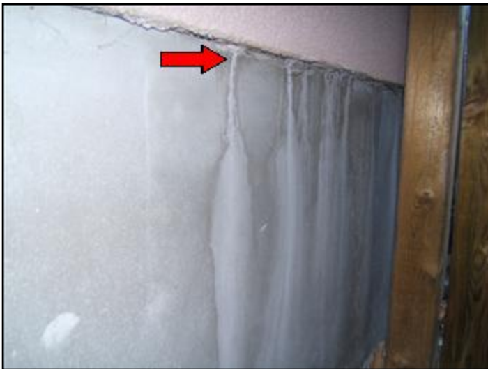
6. Possible condensation stains
